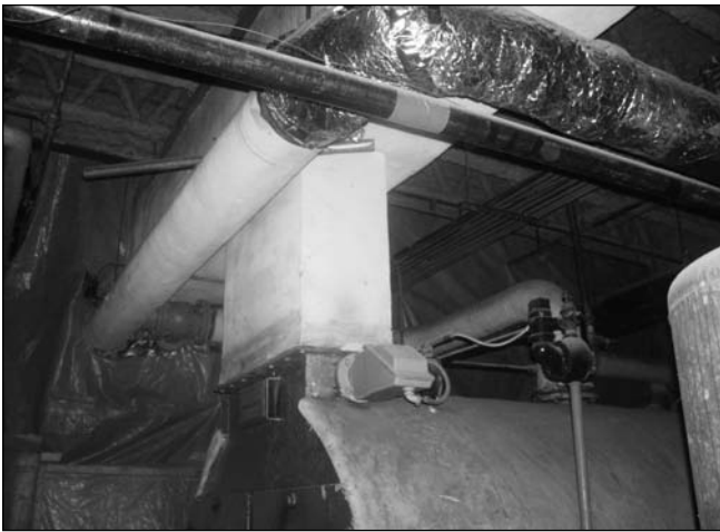
Pipe and boiler insulation
