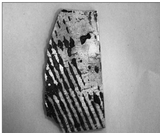
Vinyl asbestos flooring
