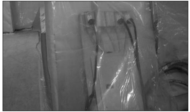
Isolated electrical panel
