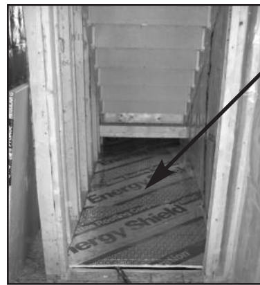
Do not restrict ventilation by blocking openings
